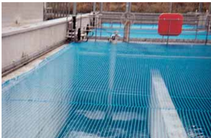
Sewage treatment safety nets
