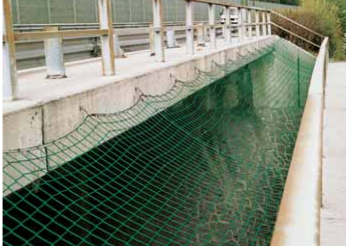
Motorway bridge safety nets
